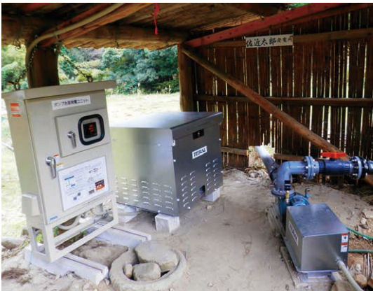
Pumping-up power generation facilities
