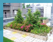
Rooftop greening system
