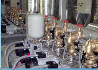
Pressurized water supply pump
