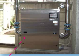
Direct connection water supply booster pump
