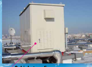
Cubicle type fire pump
